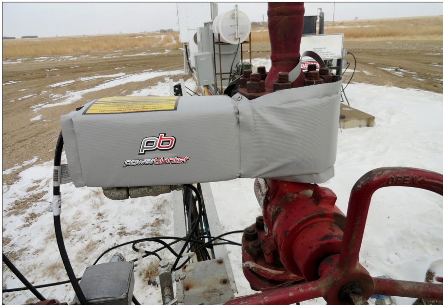
On-site Valve & Instrumentation Heater
