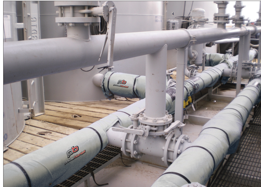
On-site Pipe & Manifold Heating System
